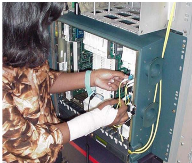
Figure 4 – Student Working With Cisco ONS 15454 System
